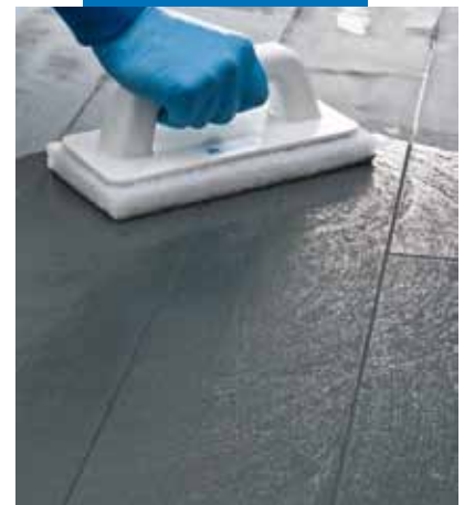
Cleaning the joints with a Scotch-Brite pad (when the product is semi hardened)
